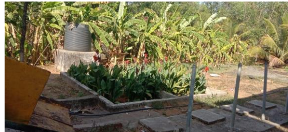
Plate 13: Faecal Sludge Treatment Plant
