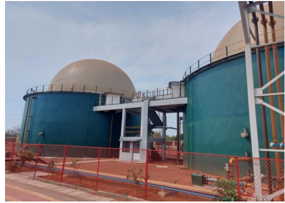
Bio-Digester for Wet Waste Processing at Saligaon, Goa
