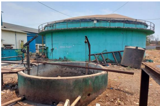
Waste to Energy Project based on Bio-Digester
