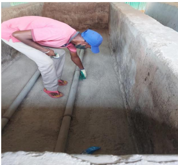
Composting Pit: - Aeration arrangement
