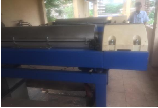
Centrifuge for sludge drying, STP Goa
