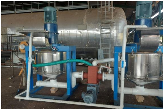
Digester for Centralized treatment of Wet Waste
