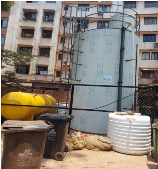
Digester for small communities – Capacity 150 Kg/day
