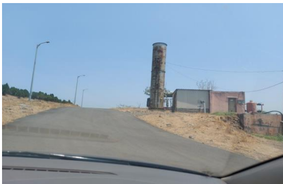
Stack for flaring bio-gas generated at Capping Site, Urali Dewachi, Pune
