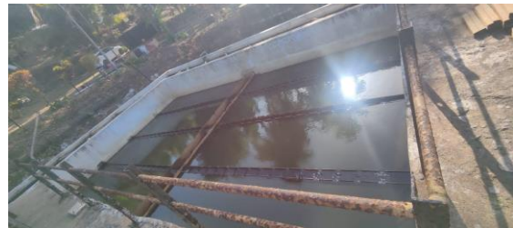
Plate 12: Water Treatment Plant : Filter
