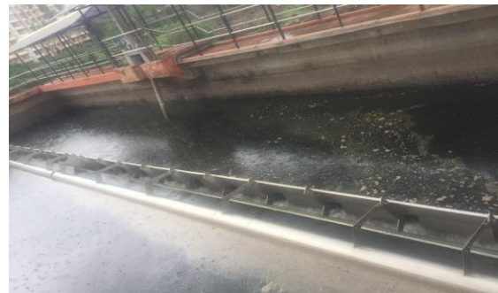
Oil & Grease Removal at STP, Goa
