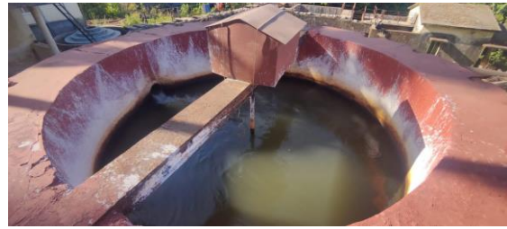
Plat No. 11: Water Treatment Plant : Cascade Aerator, Flash Mixer
